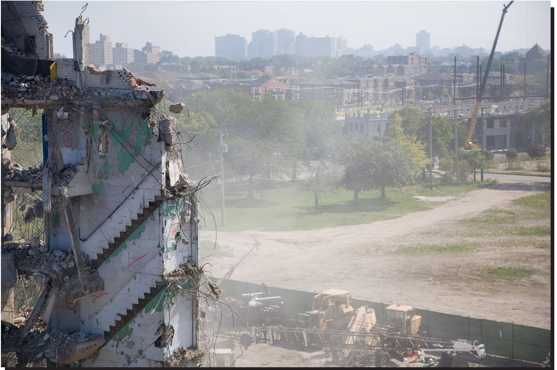
Ida B. Wells Homes Extension demolition and mixed-income development construction, 2008. Photo: David Schalliol
